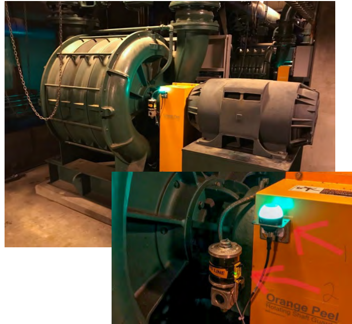
Sensors installed on 400 HP Blowers at a Veolia project. Repairs are typically $50,000 or more for just the Blower alone which made the system a value added project. The larger green bulb is the Operator touch sensor system that records date and time the oil cup was checked and the smaller green light is the oil level sensor that detects loss of oil and automatically shuts the Blower down to prevent damage.
