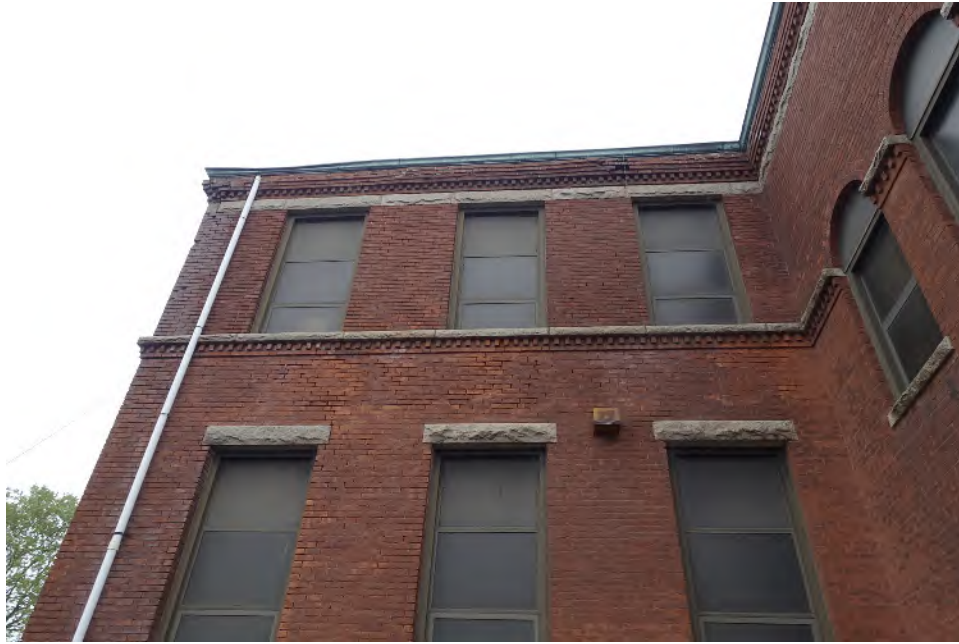
Figure 5-9. Deterioration at cornice line.
