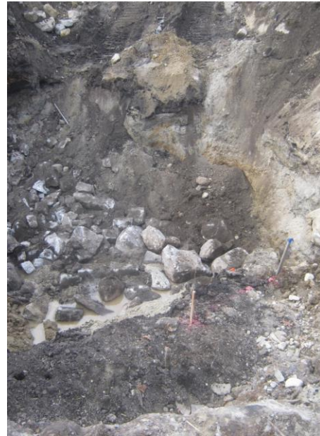
Photo 14: Backfilling PCB Remediation Waste excavation with crushed stone below groundwater table at 102 Greenwood Street on January 20, 2015.
