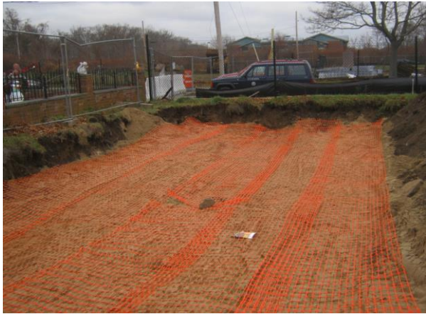
Photo 5: Orange warning layer in northwest portion of 102 Greenwood Street on December 8, 2014.
