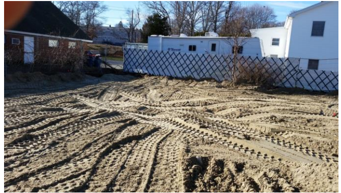
Photo 6: Majority of non-PCB Remediation Waste area of 102 Greenwood Street property graded and compacted on December 12, 2014.
