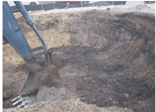
Photo 12: Removal of first five feet of PCB Remediation Waste excavation at 102 Greenwood Street on January 15, 2015.
