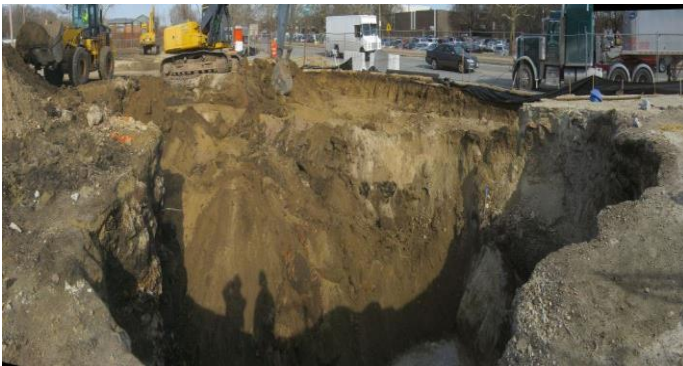
Photo 15: Using non-PCB Remediation Waste soils from zero to three feet as backfill in PCB Remediation Waste excavation at 102 Greenwood Street on January 21, 2015.
