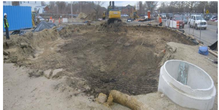
Photo 16: PCB Remediation Waste excavation at 102 Greenwood Street backfilled to three feet below grade on January 22, 2015.
