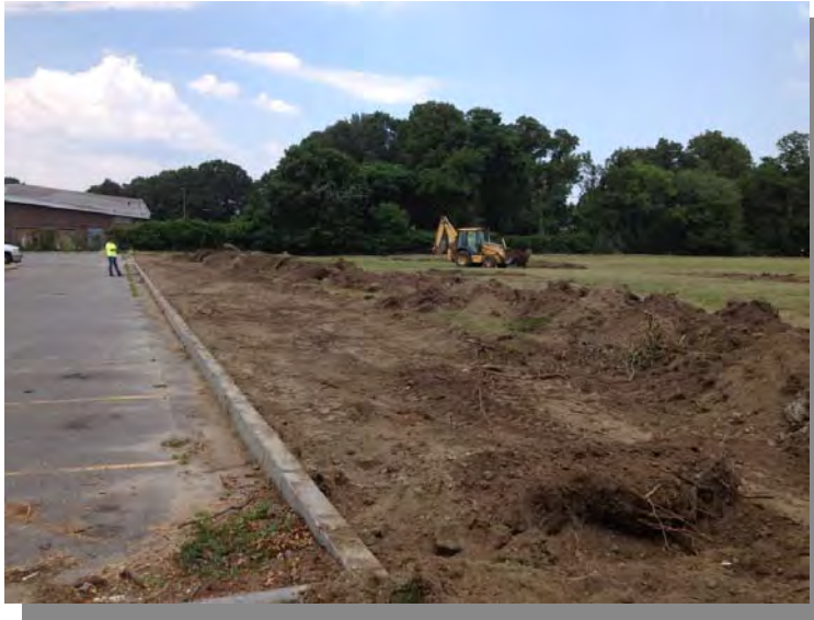
10) Excavation to 6 inches along western perimeter in support of regrading viewed to the north (7/16/13).
