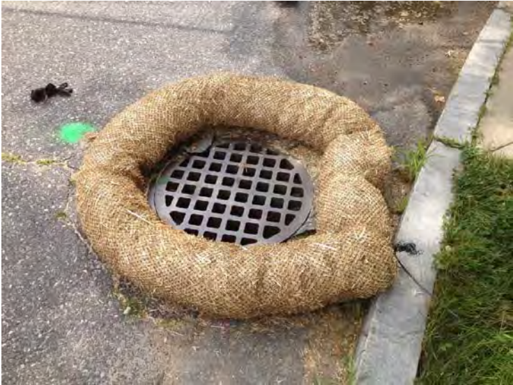
6) Catch basin erosion and sedimentation control (7/10/13).
