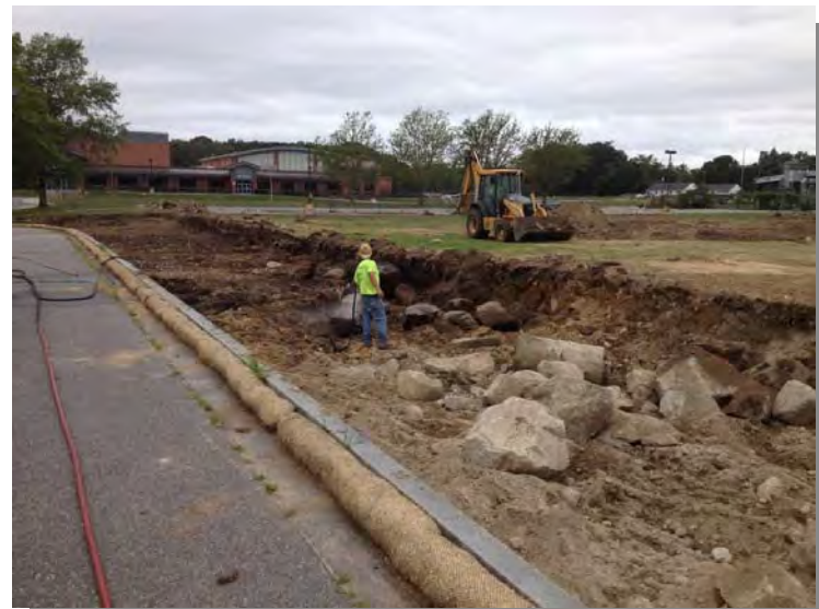
15) Pressure washing of boulders within EP HS-8 excavation viewed to the west (7/25/13)
