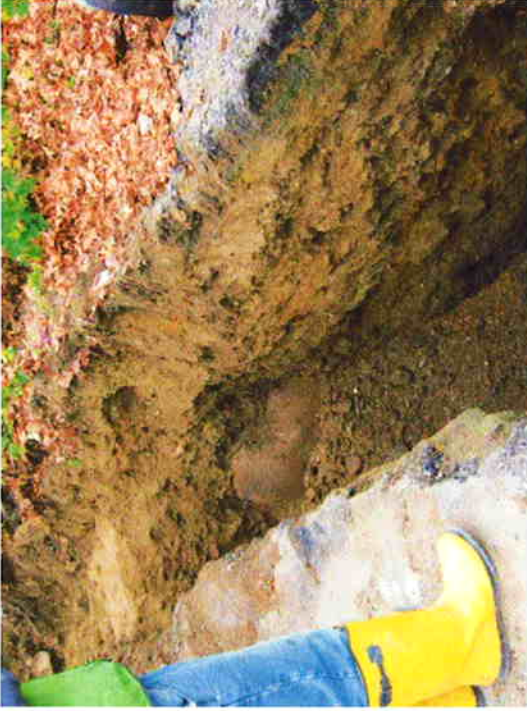
17) 48-inch diameter water main visible at edge of excavation on east side of Liberty Street (11/15/10).
