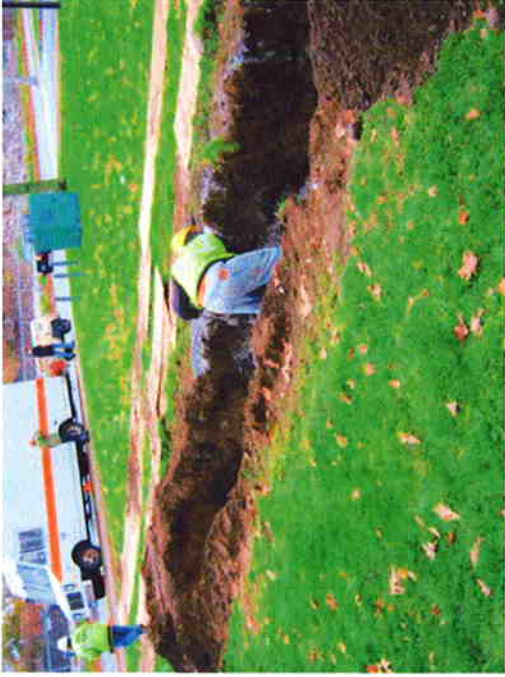
5) DPI spreading crushed stone around drainage pipe between parking lot and Liberty Street (11/9/10).
