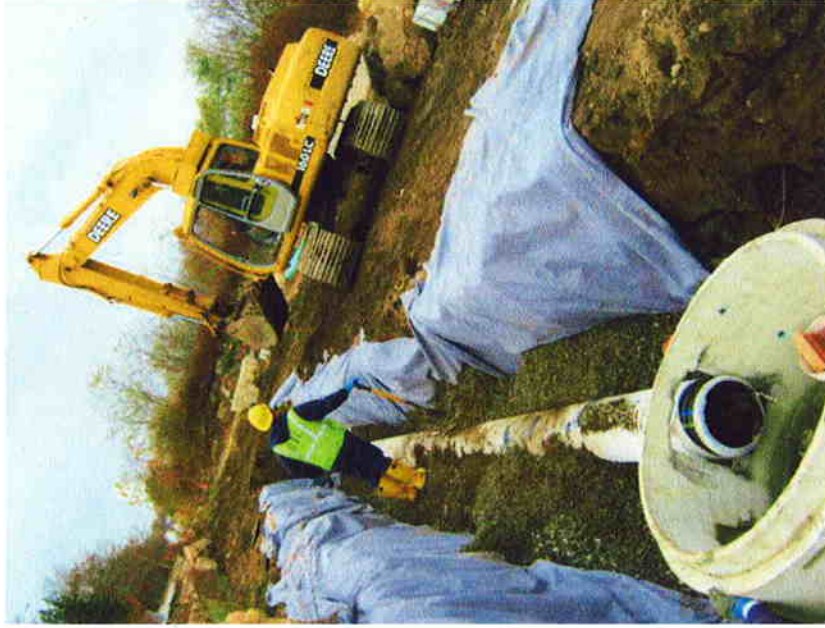
20) DPI backfilling crushed stone around perforated PVC drainage pipe along eastern side of Liberty Street (11/16/10).
