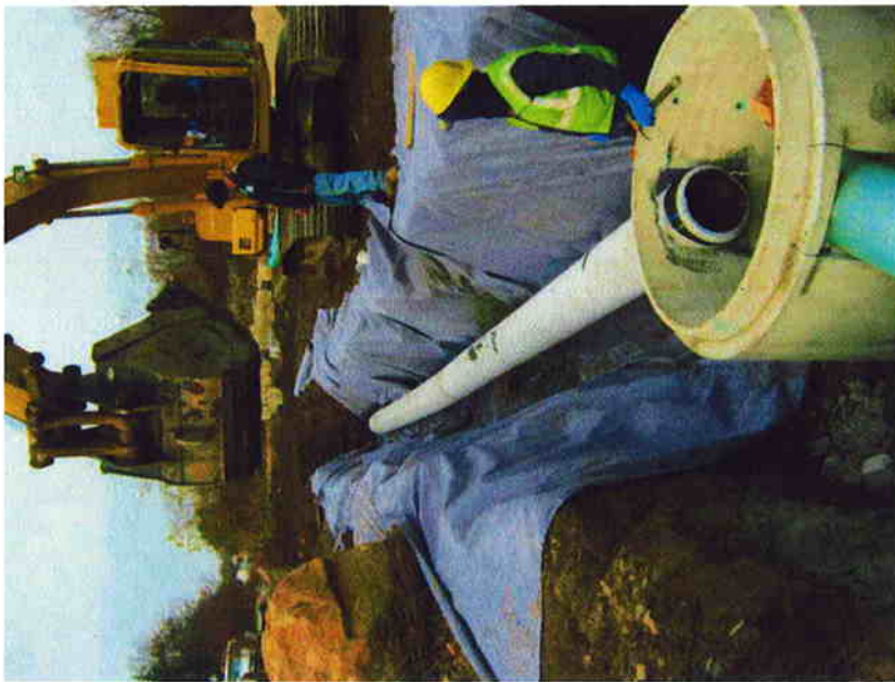
19) DPI preparing to backfill crushed stone around perforated PVC drainage pipe along eastern side of Liberty Street (11/16/10).
