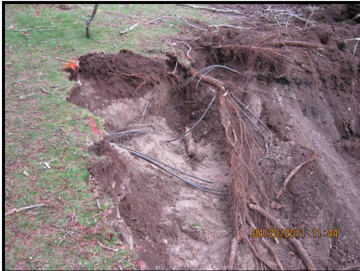
Photo 25 – Wires found in HD-20 excavation that were determined to be inactive (April 20, 2011).
