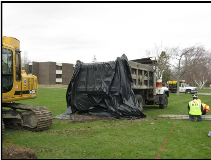
Photo 3 – Trucks lined with polyethylene sheeting while transporting soil to the Transfer Station (April 16, 2011).
