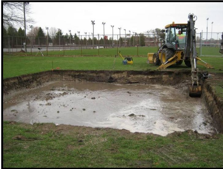
Photo 5 – Groundwater within SS-36 excavation (April 16, 2011).
