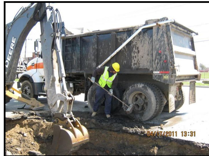
Photo 6 – Cleaning bulk soil from tires of truck before leaving the work zone (April 17, 2011).
