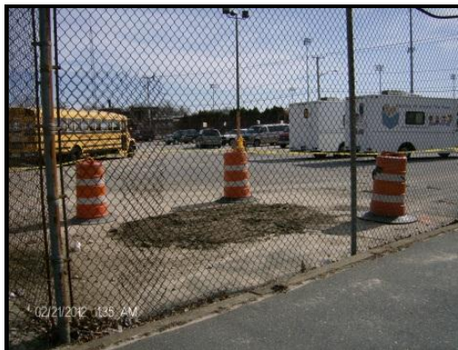
Photo 3: Excavation area within the northwest corner of the Bus Yard (view from the northwest) with Parker Street in the background.
