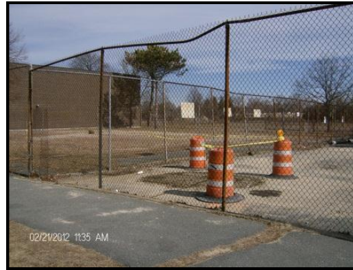
Photo 2: Excavation area within the northwest corner of the Bus Yard (view from the southwest).
