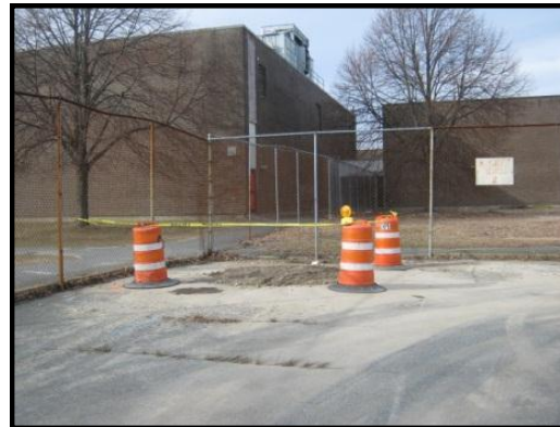
Photo 4: Excavation area within the northwest corner of the Bus Yard (view from the south) with NBHS in the background.
