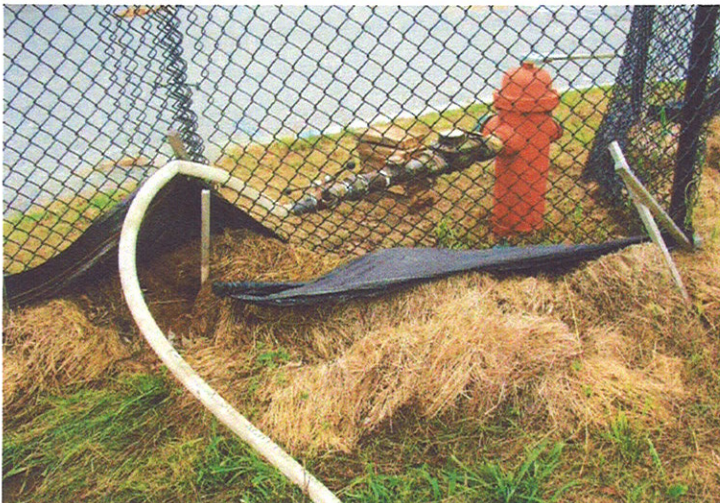
3. Readily available water for dust suppression from hydrant on the corner of Hathaway Blvd. and Ruggles Street (7/15/10).
