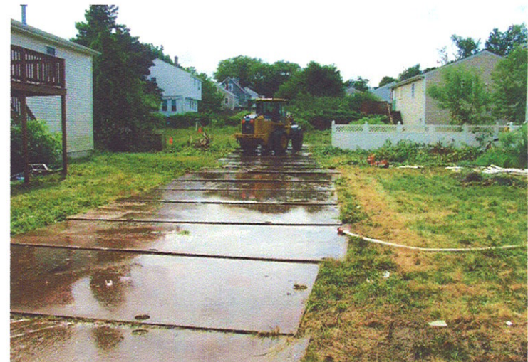
2. Steel plate road down center of Site to avoid contact with soil (7/15/10).
