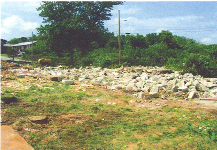
15. Broken concrete foundation walls and basement slab material at 108 Ruggles Street (7/24/10).
