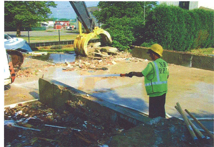
6. Structural debris removal at 102 Greenwood Street. Concrete intact and to be crushed and hauled offsite (7/19/10).
