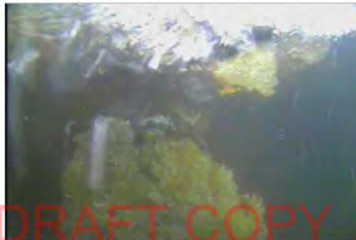
Photograph 8: Bent 15 Pile C2 - complete loss of flanges
