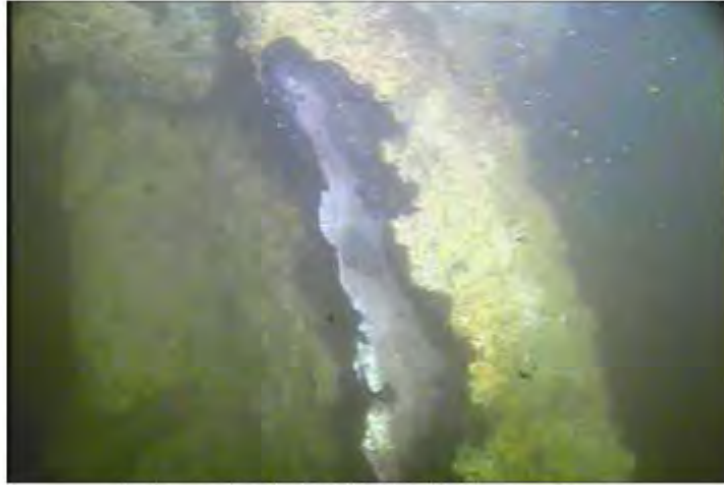
Photograph 9: Bent 16 Pile 16.3 2 - flange edge
