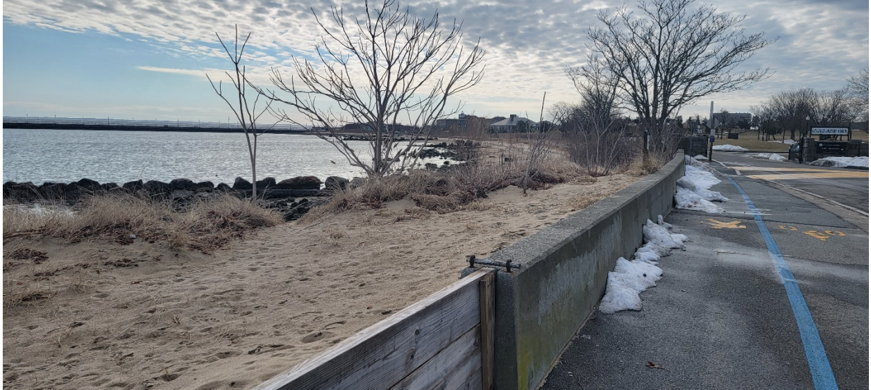
Photo 13: South view of Coastal Dune (continuing from Photo 12), vertical concrete sea wall (with wooden barrier at an opening for pedestrian access), and bike path to the east of East Rodney French Boulevard.
