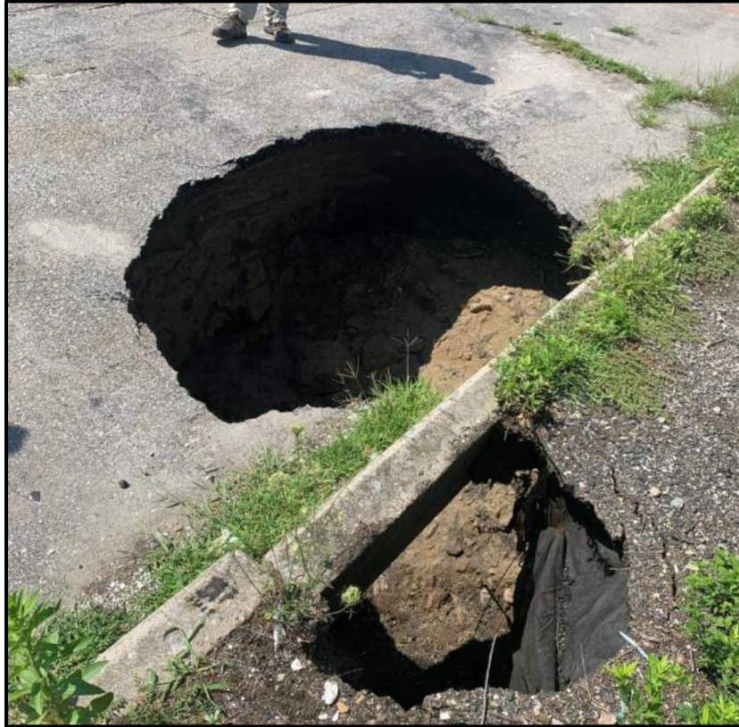
Photograph 1 – MassCEC Terminal Sinkhole
