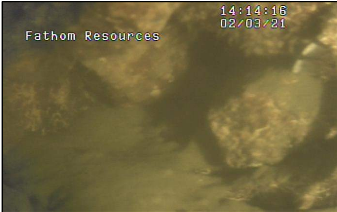
Photograph 3 – Shuster Bulkhead Washout Below Steel Sheet Pile
