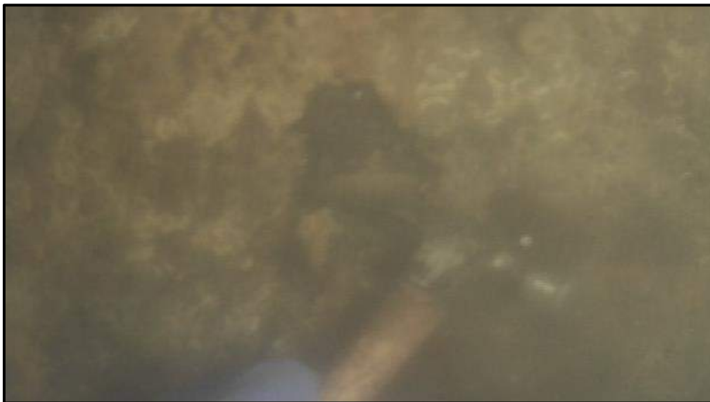
Photograph 2 – Shuster Bulkhead Typical Hole in Sheet Pile Wall
