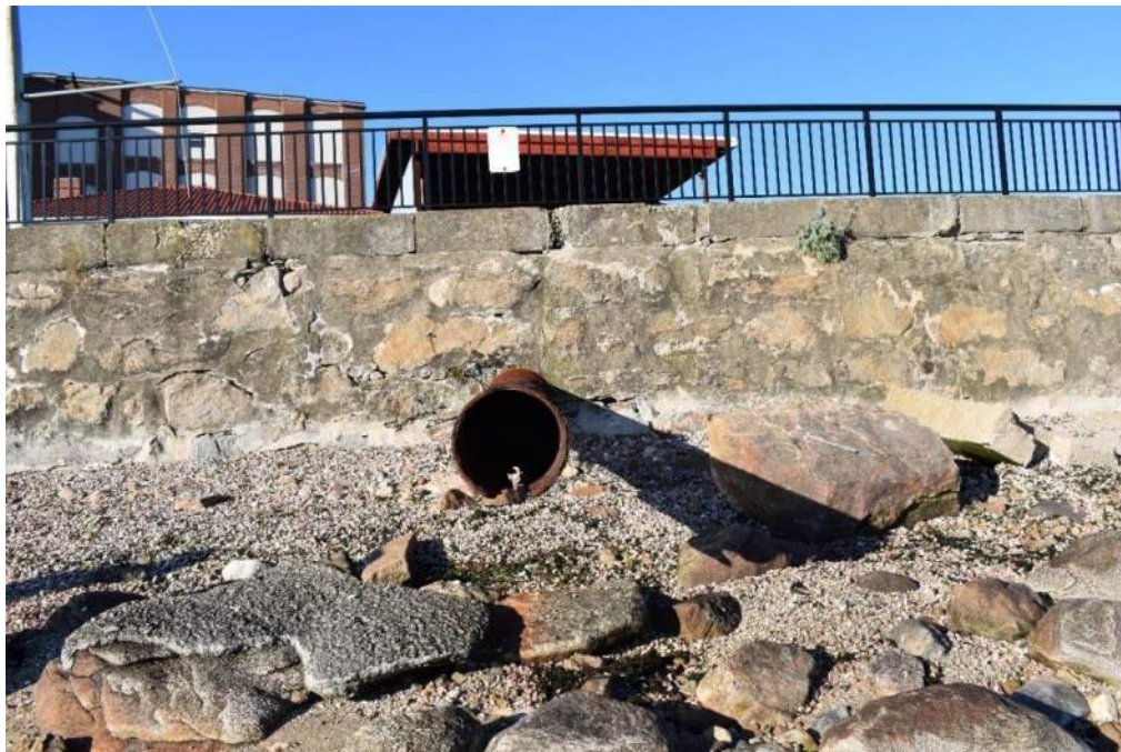
Photo 8: Outfall pipe near the Irish Monument in poor condition
