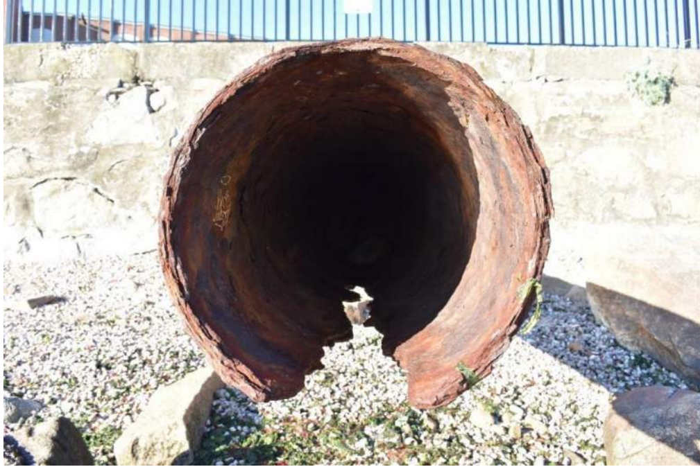
Photo 9: Outfall pipe near the Irish Monument in poor condition
