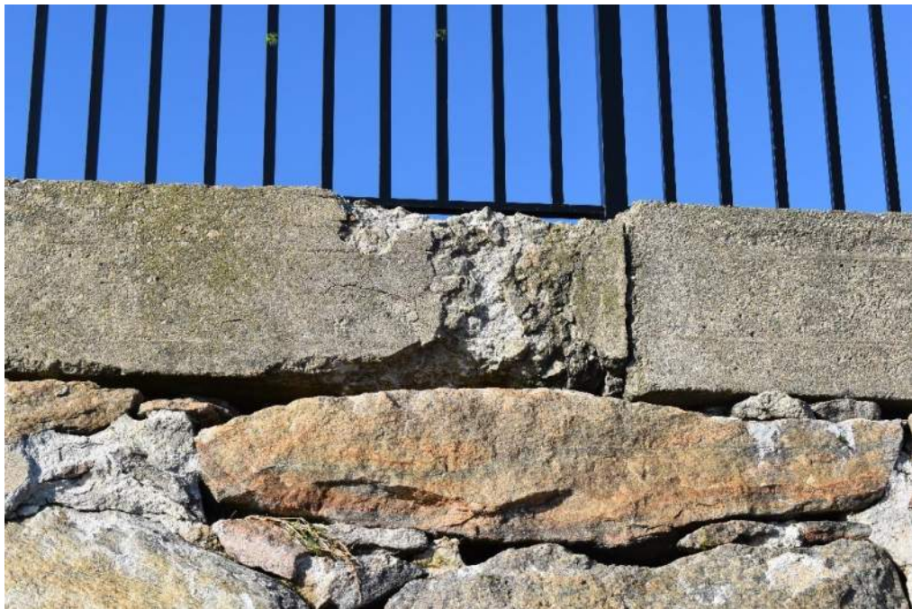
Photo 12: Concrete Cap in poor condition
