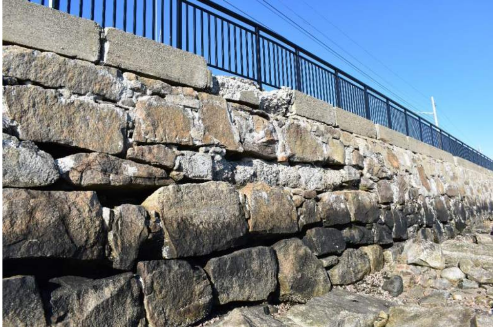
Photo 15: Concrete Cap in poor condition
