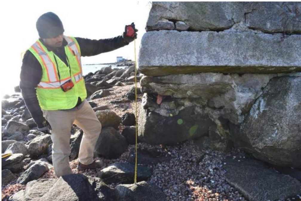
Photo 4: Missing block at the corner of the Irish Monument
