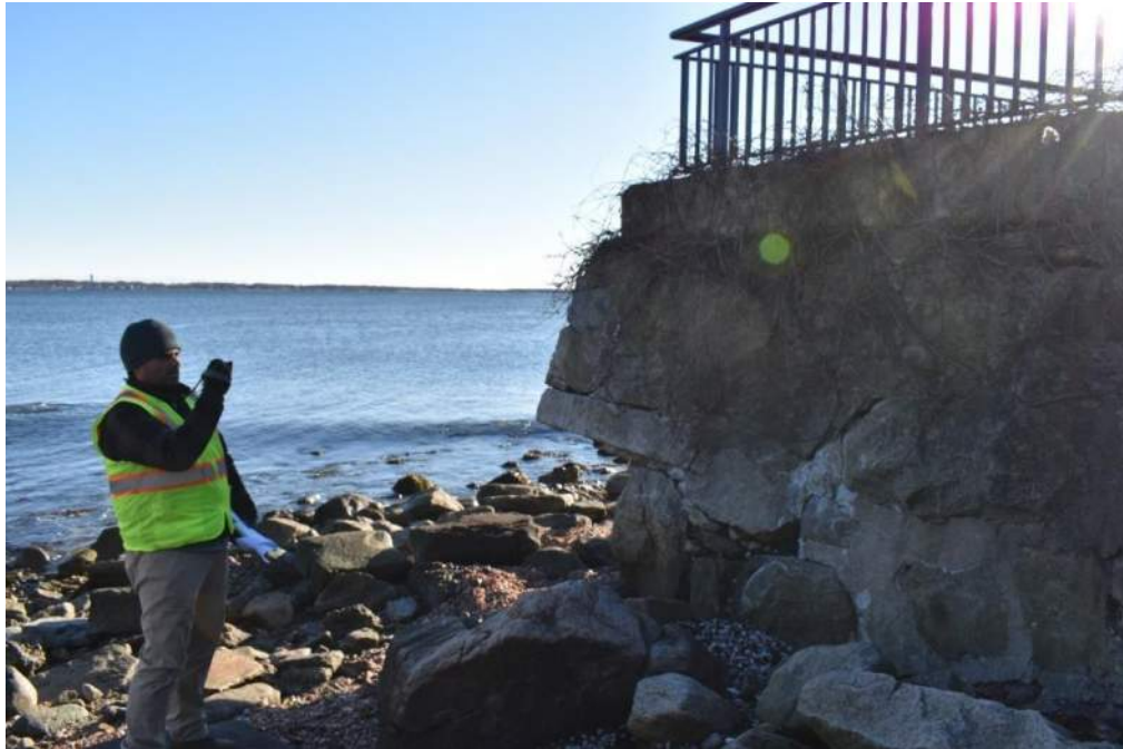
Photo 5: Missing block at the corner of the Irish Monument
