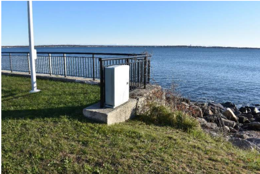
Photo 1: Most southern portion of the seawall at the Irish Memorial Monument, looking East.
