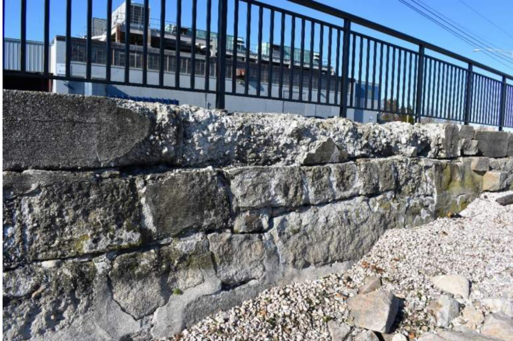
Photo 21: Concrete cap in poor condition
