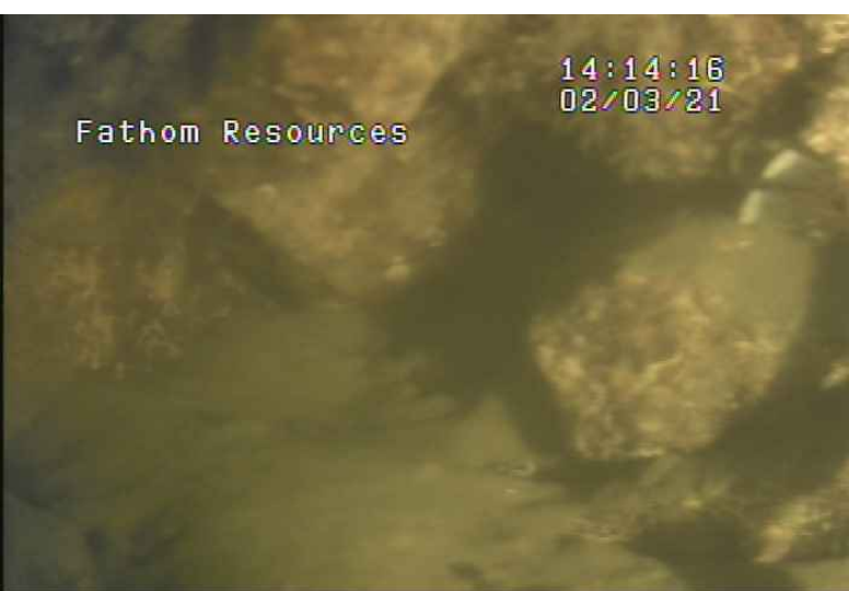
CELL #6: SHEETS SITTING ON ROCKS W/ LARGE VOID SPACE BENEATH SHEETS; WASHOUT OCCURRING BELOW OLD BRIDGE DEPTH LIMIT
