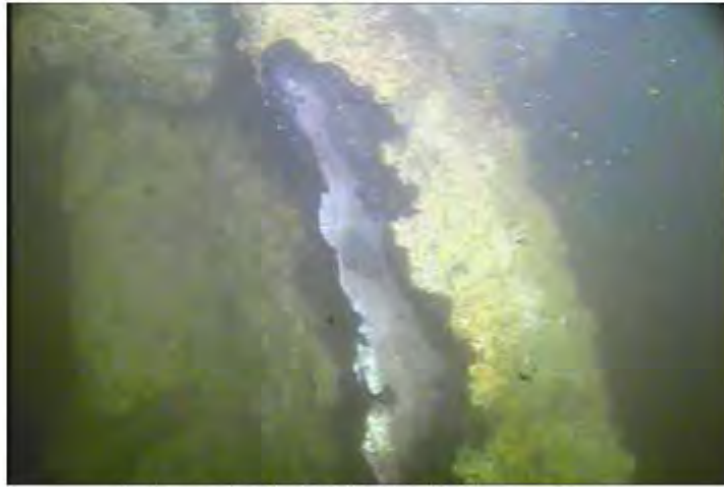
Photograph 9: Bent 16 Pile 16.3 2 - flange edge
