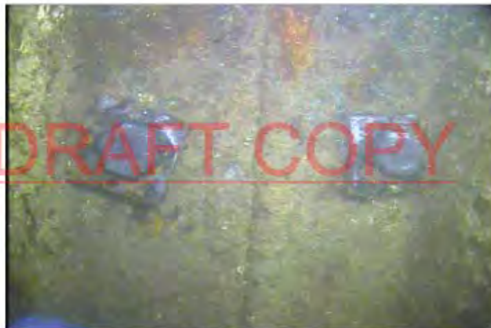
Photograph 12: Tieback bolts through bulkhead
