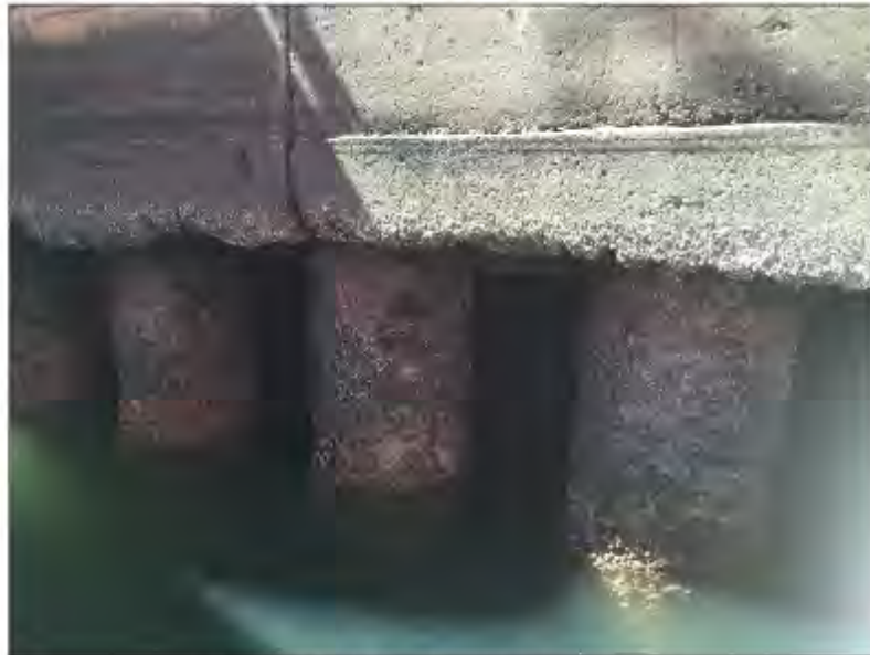
Photograph 2: Typical close spacing of piles
