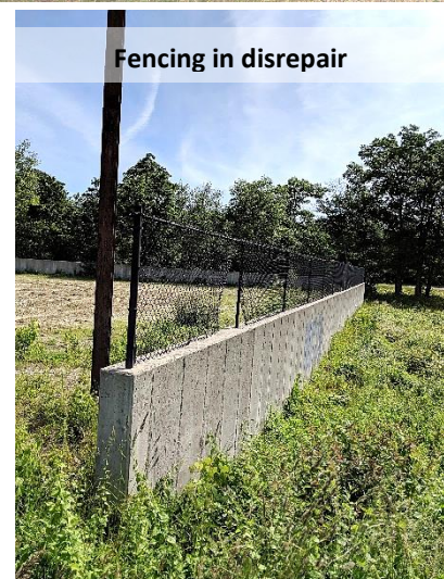
Fencing in disrepair
