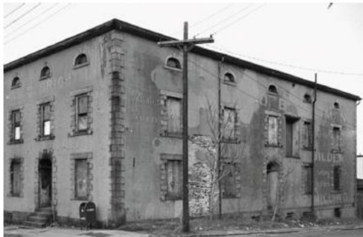
The Rodman Candleworks Building, having fallen on rough times. Photo, from Spinner Books.
