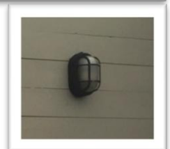
Current wall sconces
