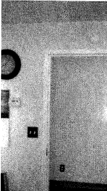
7 Provider Office 2, Smoke detector
