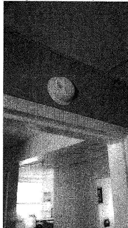
8 Provider Office 3, Smoke detector
