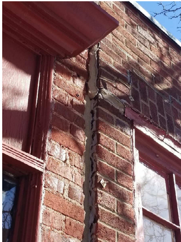
Photo #12 – Masonry wall pulling away from the front of the structure approximately 2".
