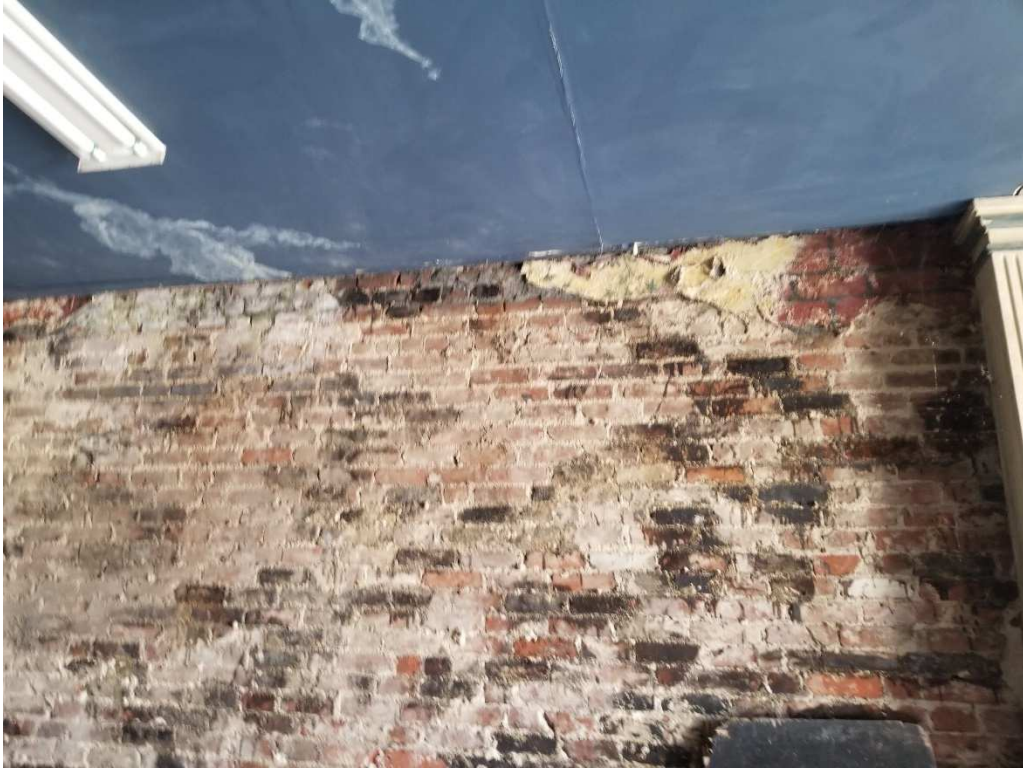
Photo #9 – Water intrusion at the back wall.
