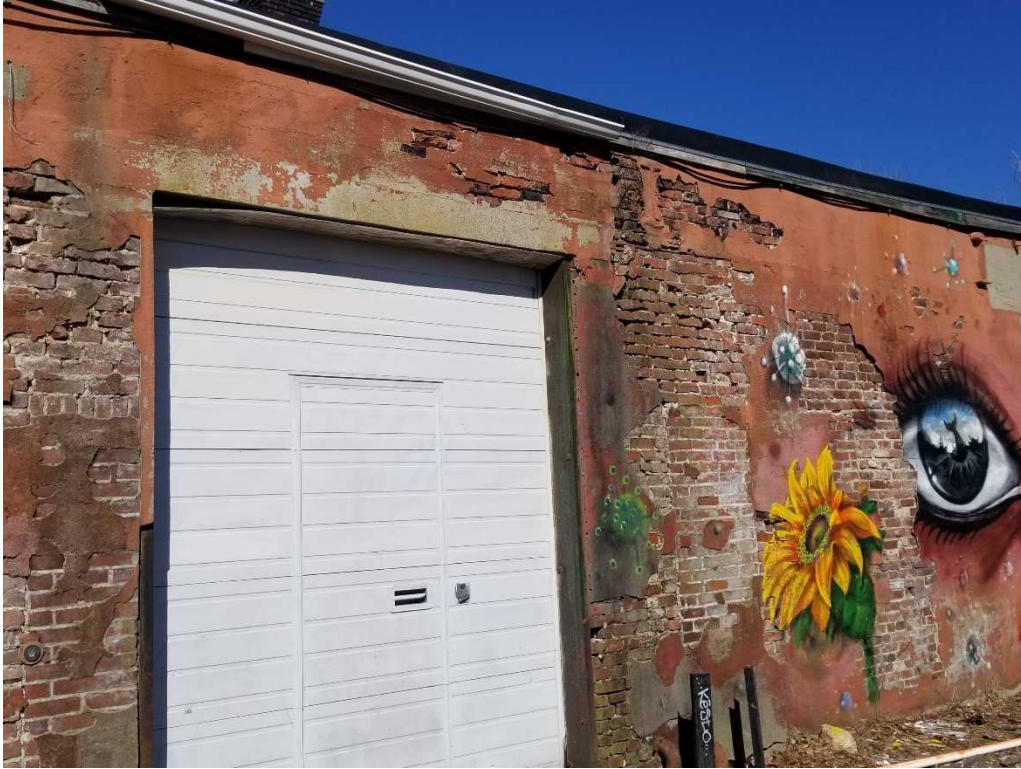
Photo #19 – Gutter above overhead door with no downspout.
