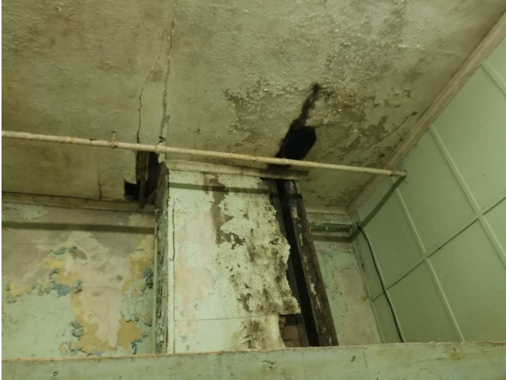
Photo #23 – The wood framing is deteriorated and starting to collapse.
