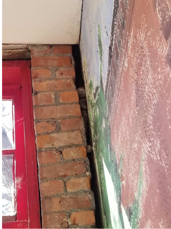
Photo #11 – Daylight can be seen from the masonry pulling away from the structure.
