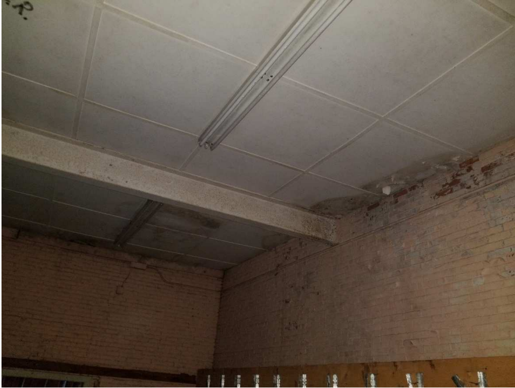
Photo #17 – Water intrusion at the front of the building, adjacent to 121 Union street.
