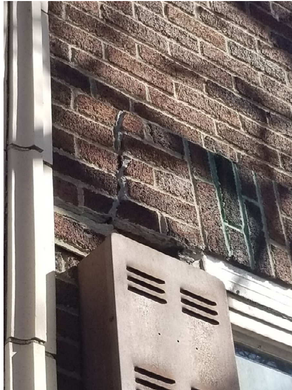
Photo #5 – Façade pulled away from the building approximately 1”.
