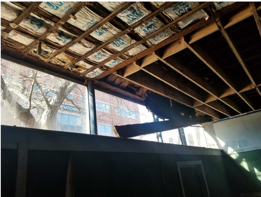
Photo #2 – Steel girder, perimeter steel lintel assembly and wood framing deteriorated at front façade.
