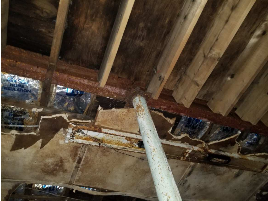
Photo #7 – Steel girders and columns severely deteriorated.
