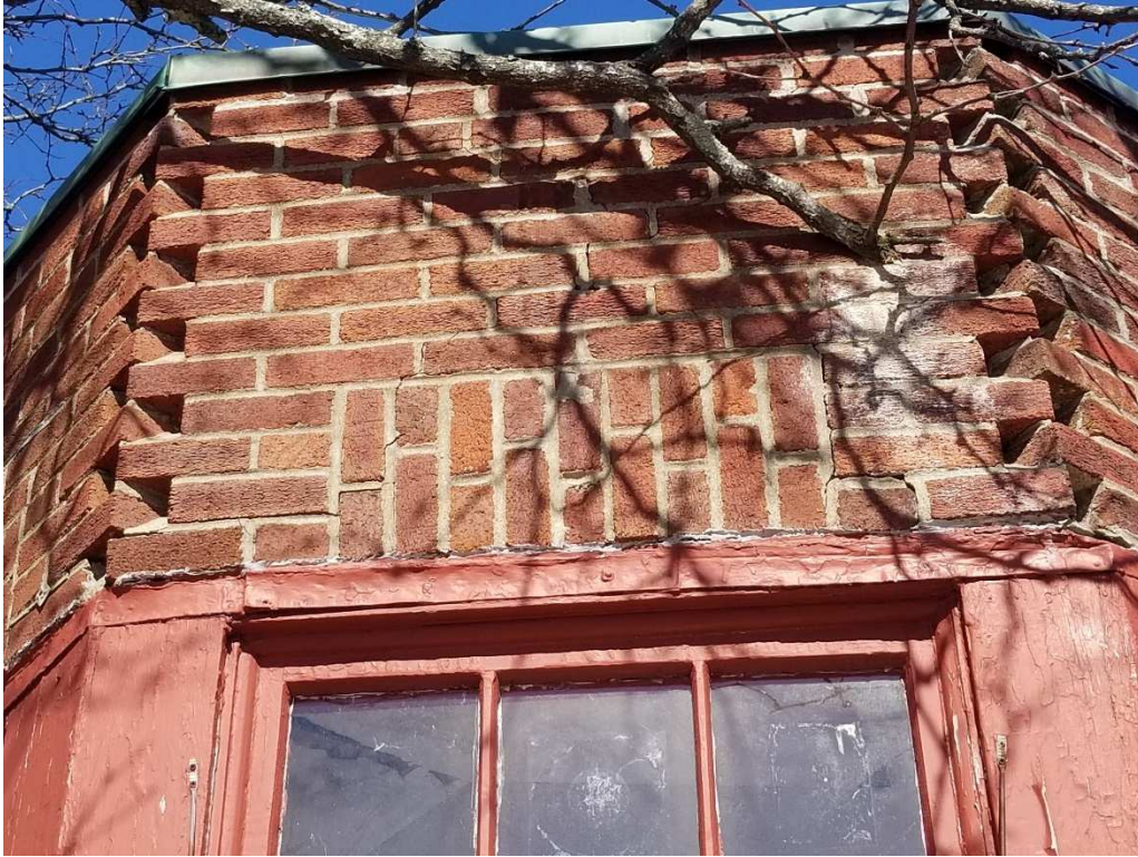
Photo #15 – Diagonal cracking above front lintel assembly.
