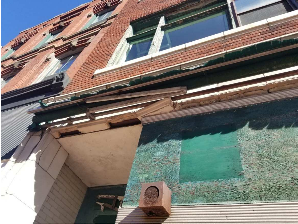
Photo #21 – Masonry band is deteriorated and spalling off the building.
