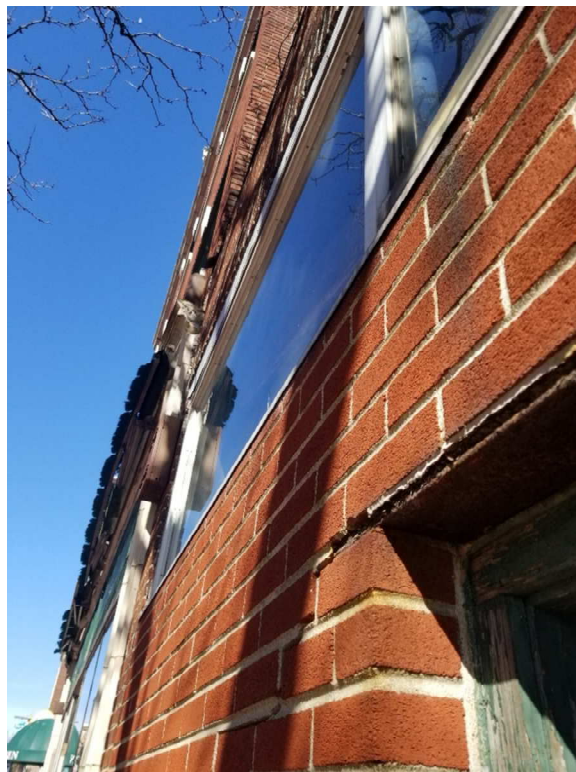
Photo #6 – Façade pulled away from the door lintel approximately 1”.
