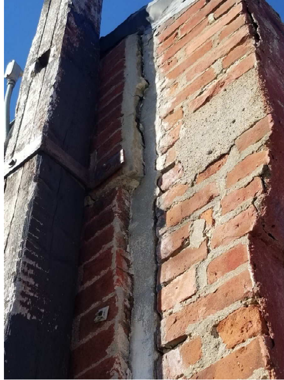
Photo #13 – Masonry wall pulling away from the back of the structure approximately 2”.
