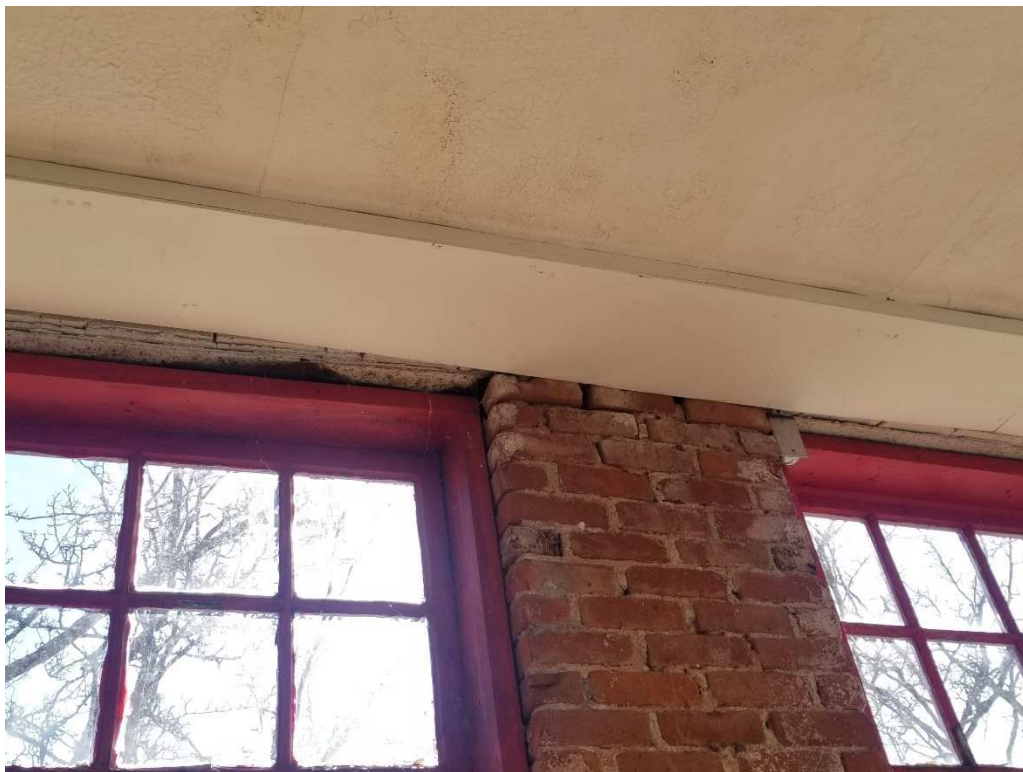
Photo #14 – Lintels excessively deflecting and the masonry deteriorated at the supports.
