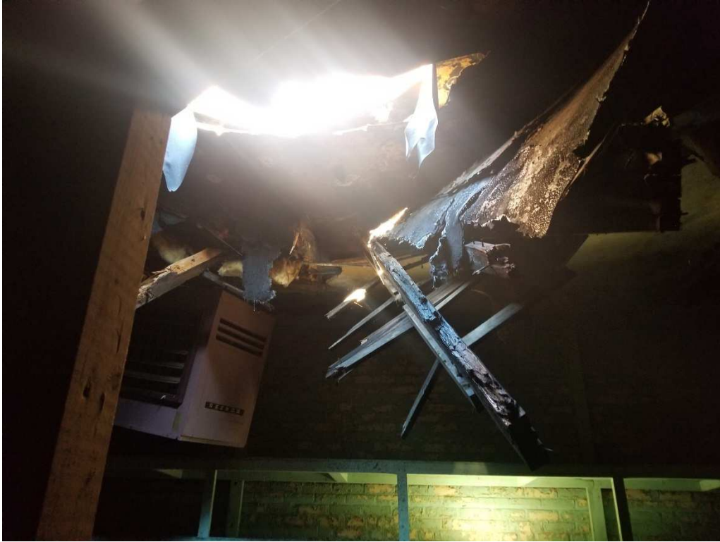
Photo #1 – Roof collapse at the back of the building adjacent to the 3-Story Building.
