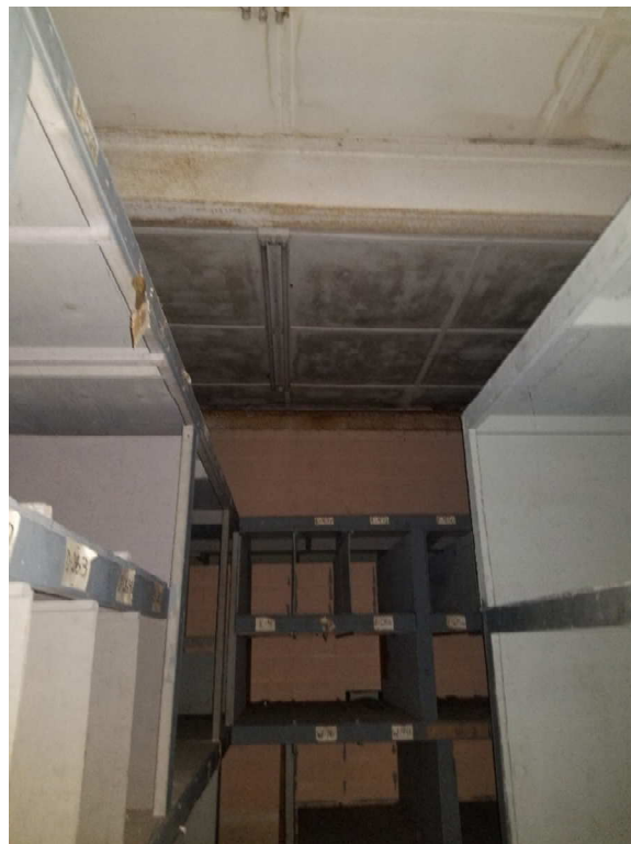
Photo #18 – Water intrusion at the back of the building.
