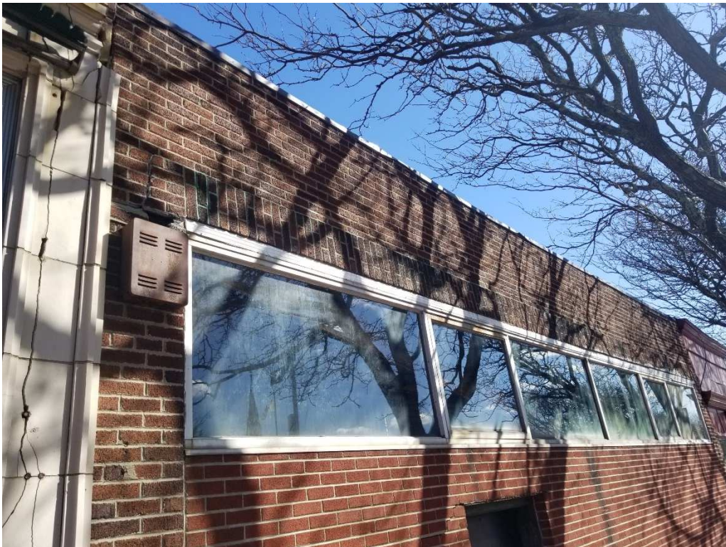
Photo #4 – Front façade pulling away from the building at the failed lintel assembly.
