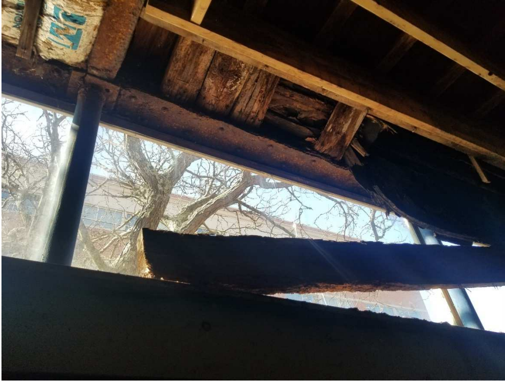
Photo #3 – Steel girder, perimeter steel lintel assembly and wood framing deteriorated at front façade.
