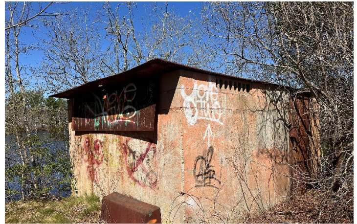
Abandoned pump house. At the north of the property along the south side of the pond.
